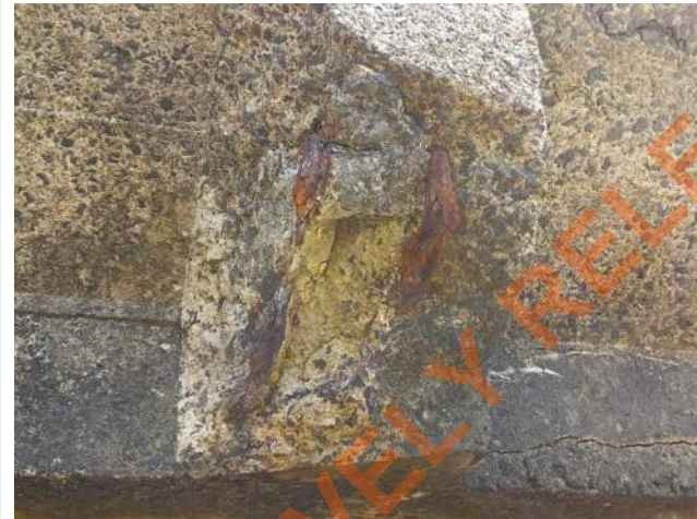
Spalling of concrete with Existing transverse bottom reinforcement lost due to severe corrosion.
