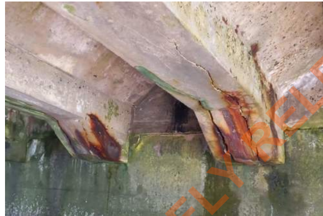
10mm- 20mm significant Longitudinal concrete cracks along existing P.C beams with severe induced corrosion of reinforcement bars.
