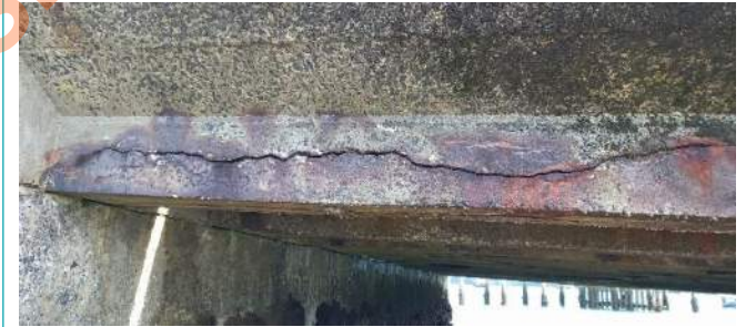
15mm- 22mm significant Longitudinal concrete cracks along existing P.C beams with severe induced corrosion of reinforcement bars.
