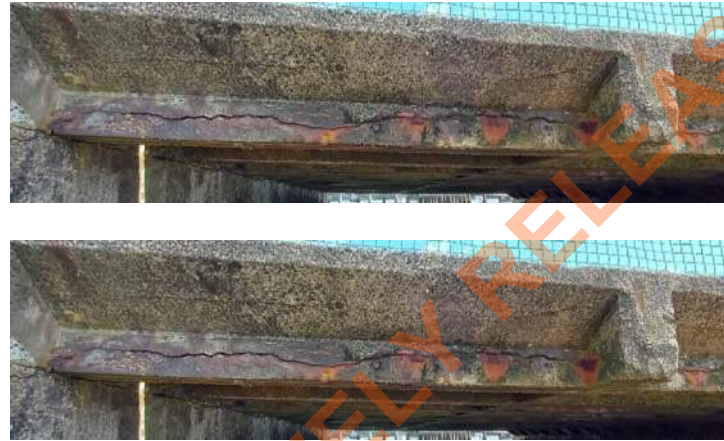
10mm- 20mm significant Longitudinal concrete cracks along existing P.C beams with severe induced corrosion of reinforcement bars.
