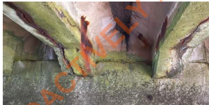
10mm- 20mm significant Longitudinal concrete cracks along existing P.C beams with severe induced corrosion of reinforcement bars.
