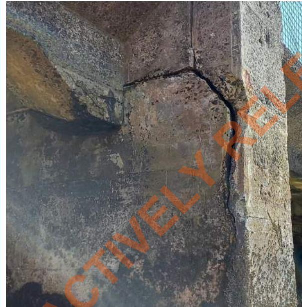
Severe concrete cracking of the capping beam upstand at the eastern end, approx 20mm wide.
