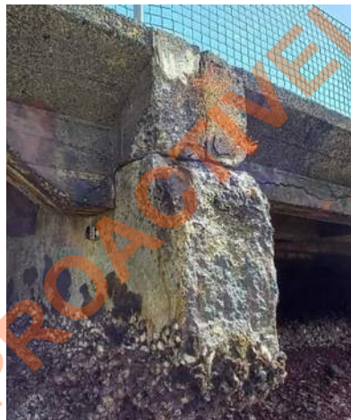
Capping beam eastern end upstand wall lost due to severe concrete spall and reinforcement corrosion.
