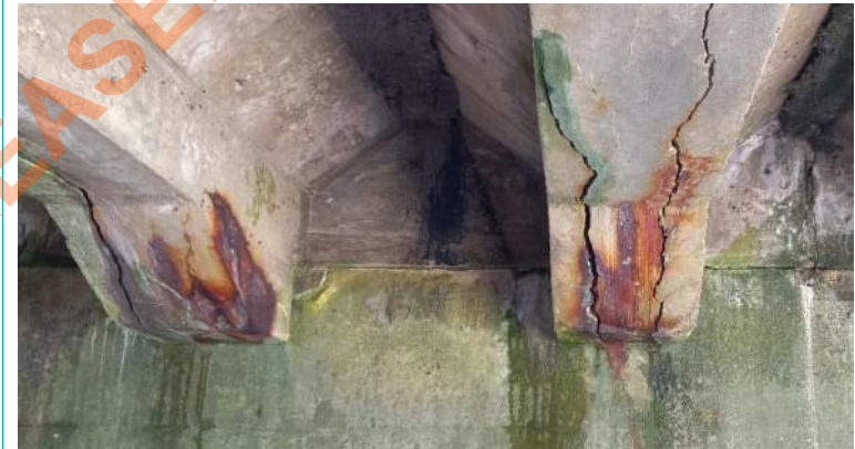
15mm- 23mm significant Longitudinal concrete cracks along existing P.C beams with severe induced corrosion of reinforcement bars.
