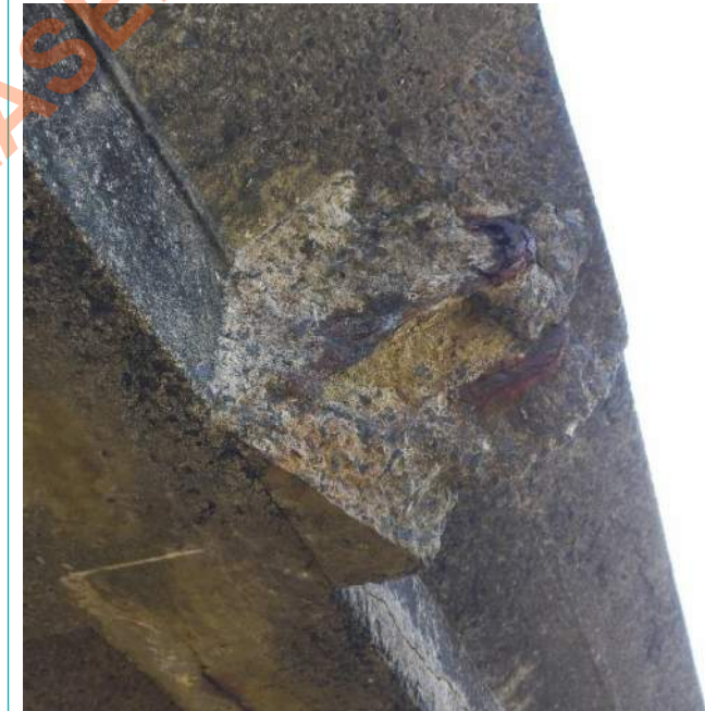
Existing transverse bottom reinforcement lost due to severe corrosion
