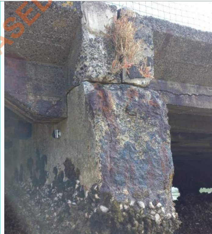
Capping beam eastern end upstand wall, severe corrosion induced cracking of concrete.
